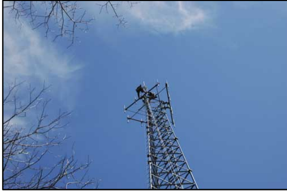
Berkshire Wireless installing equipment on cell tower in Warwick. Photo courtesy of Ray Lemek.
