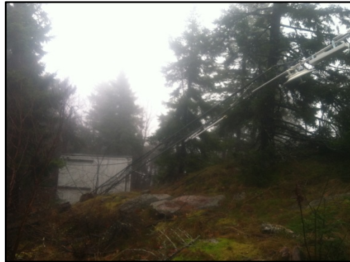
Downed communication tower in New Hampshire. Photo courtesy Brian Foucher at Wivalley.net.
